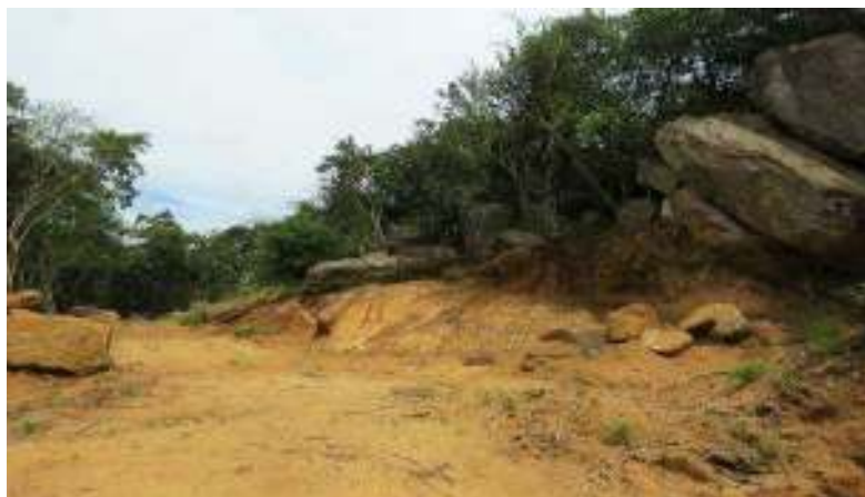
Figure 169 Soil erosion from cleared lands and excavated soils as well as slope instabilities in hill slopes take place. Loss of the stability of fractured and loosed rock slabs within the hill slopes of dam abutments
